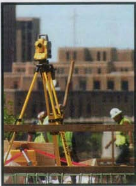
A Trimble 5603 Total Station is set up on the bridge deck near the north abutment of Pier 4.
